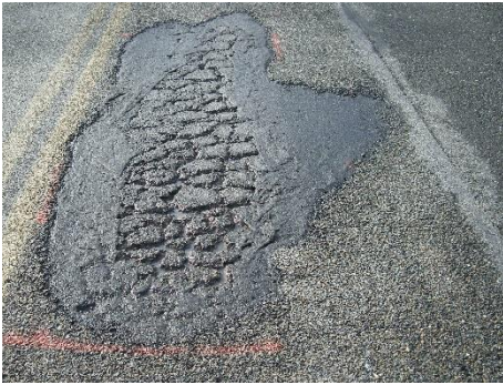
Figure 3 Petromat Failure on Crystal Blvd
